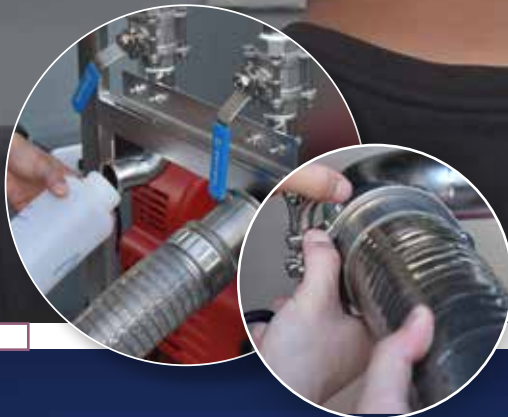
Permeate pipes with ball valves allow for easy sampling during system operation.
